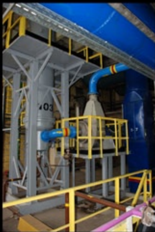
(Top) Steel equipments framework, steel platforms.
