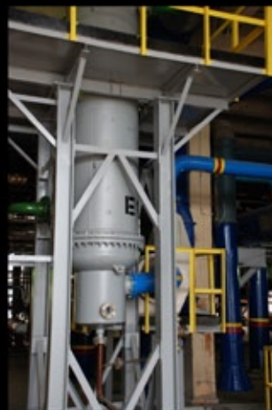
(Top) Steel equipments framework, steel platforms.
